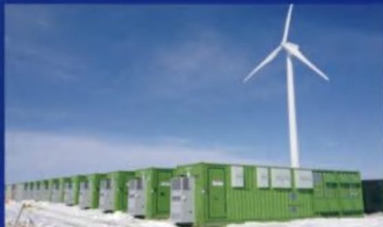
储能系统 Energy storage
